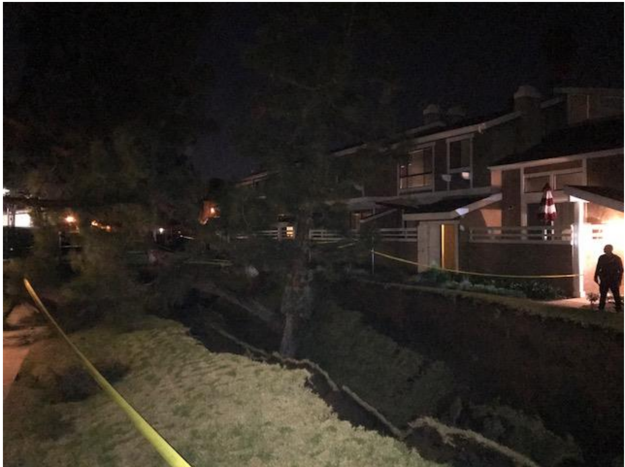
Flood control channel collapses causing a large sink hole.
